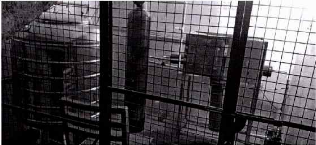
RO Water Plant
